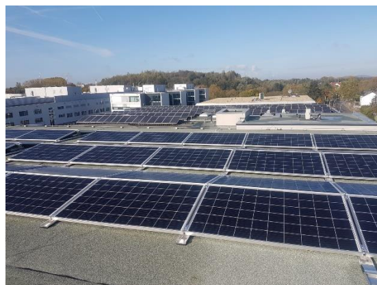
Photovoltaic installation on our buildings
